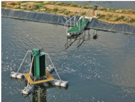
New low carbon footprint Aero-Fac® Treatment Works at Roundwood replaced old filter works.
