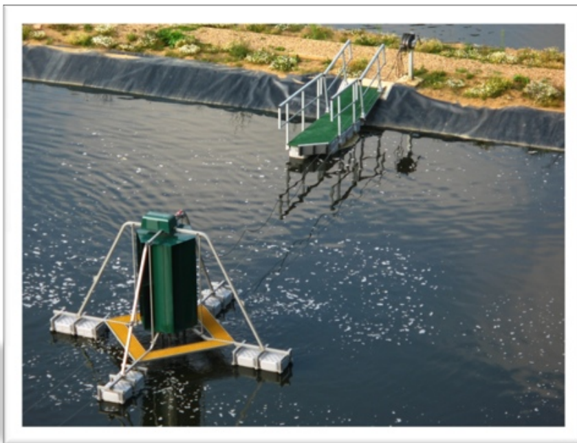
Photo 3 — The Series 3 windpowered aeration units provide zero-to-low cost aeration and optimisation of the facultative process.
