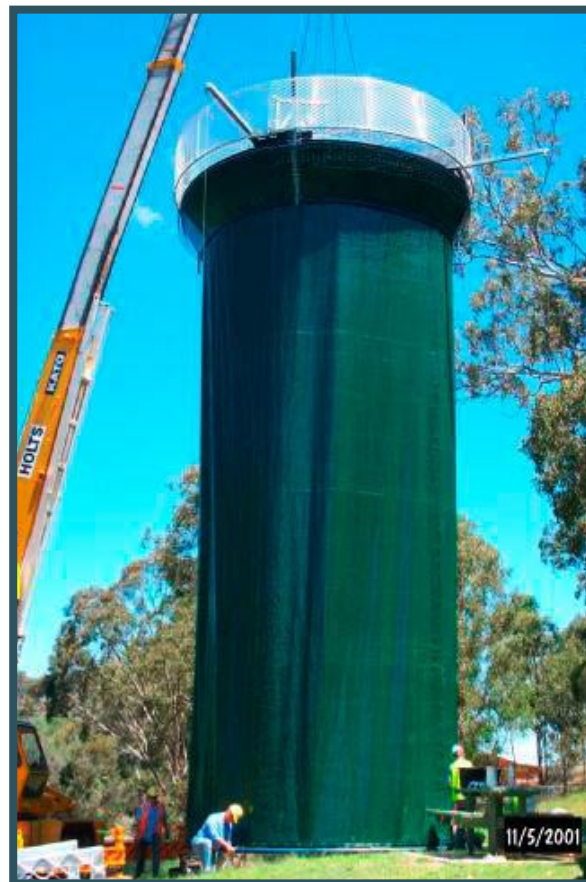
Figure 9. One of the WEARS SMDI-5s, to be coupled with another, being prepared for installation at Cooby Dam for the Toowoomba City Council.
